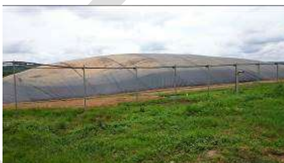
1000m 3 biogas reactor © RETT Project
