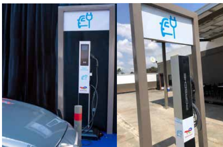
Figure 9: TotalEnergies Charging Station located Near 37 on the Liberation Road
