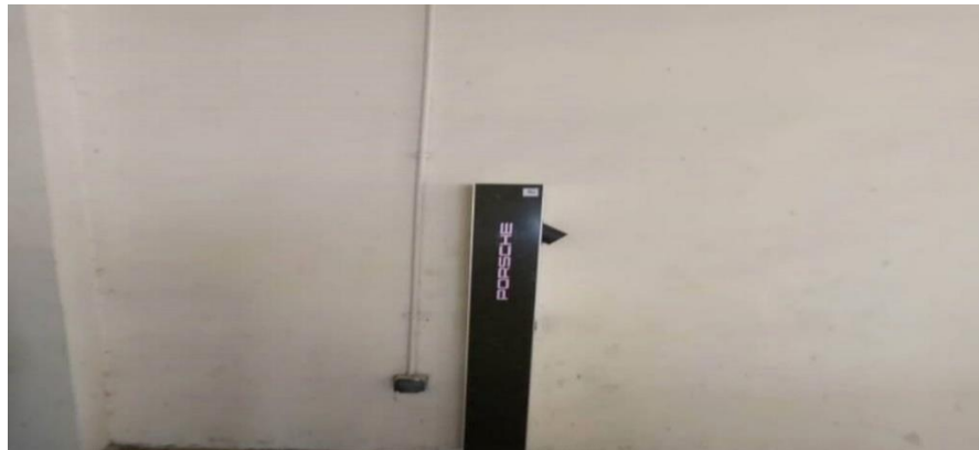
Figure 8: Porsche Charging Station located at Kempinski Hotel
