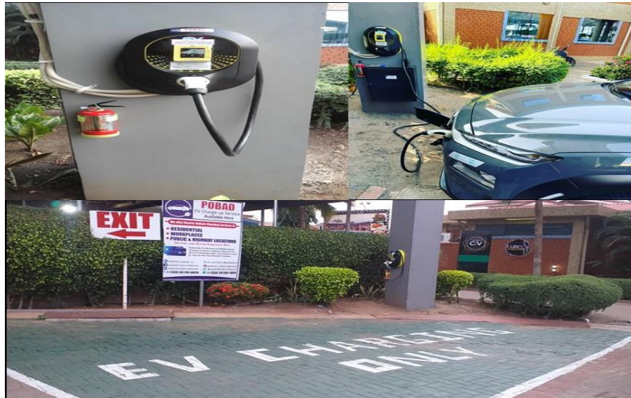
Figure 6: POBAD Charging Station Located at the A&C Mall, East Legon
